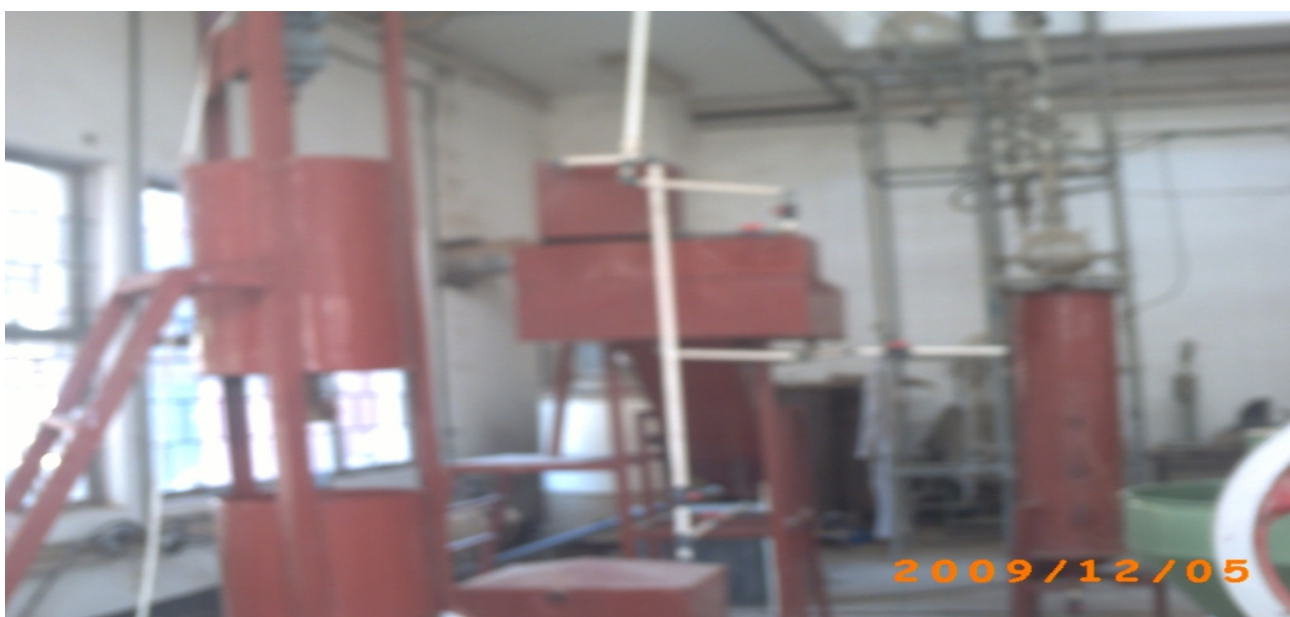
Figure 2. A Pilot Plant for Water Treatment showing the Major Unit Processes and Operations
