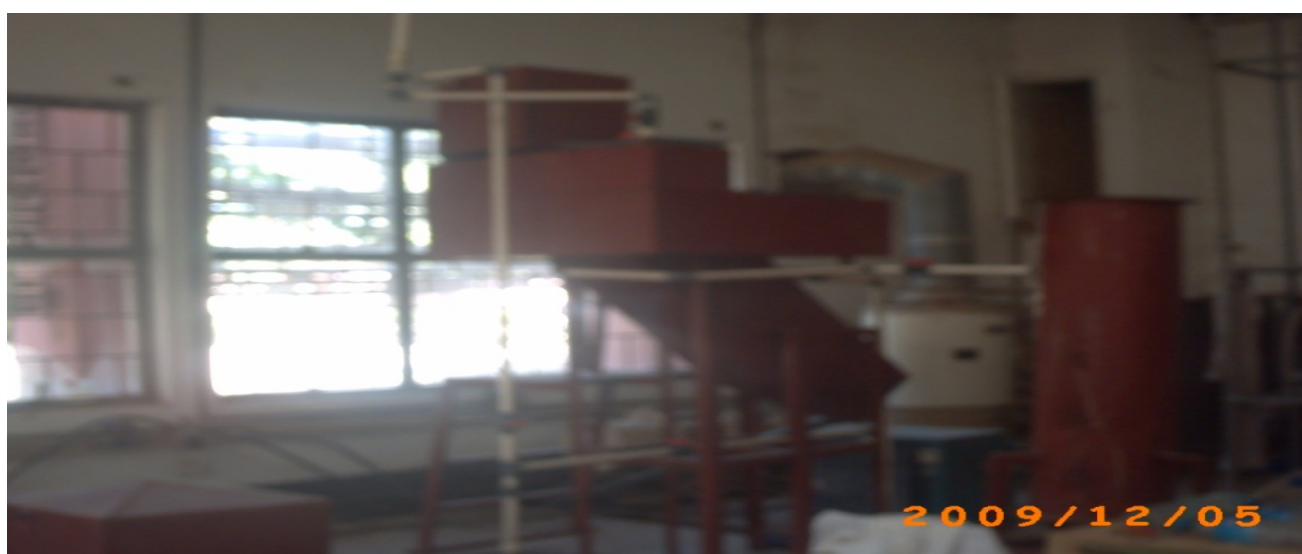
Figure 3. A Pilot Plant for Water Treatment showing the Coagulation, Flocculation, and Sedimentation Processes
